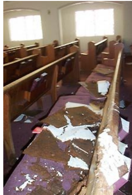
The sanctuary of First Baptist Church in Raymondville was trashed by Hurricane Dolly. (photo courtesy of the imlivingoutloud blog by Kathy Carlton Willis)
