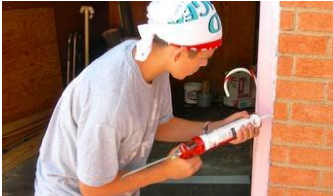
Christian Leonard, 14, takes care to seal crevices with caulk along brick of a home in Dallas. (PHOTOS/Grace Gaddy)
