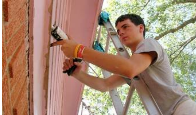
Josh Kicker, 14, uses a caulk gun for sealing as he works on a World Changers project in Dallas. (PHOTOS/Grace Gaddy)
