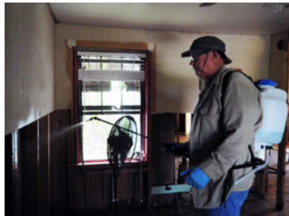
Butch Abernathy, a Texas Baptist Men volunteer from Oak Grove Baptist Church in China Spring, sprays surfaces of a flood-damaged home in Sonora to mitigate mold. (Photo / Ken Camp)
