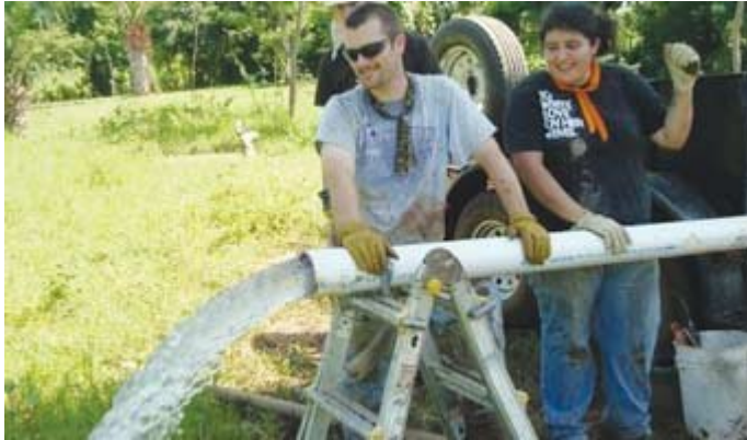
Steadying a pipe as water first comes out are Derek Dodson (left), BSM director at Tarleton State University, and Cheli Urquiza, a junior communications major at Angelo State University.
