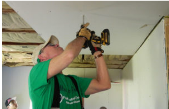
Steve Carter from First Baptist Church in Norman, Okla., installs drywall on the interior ceiling of a storm-damaged home in Refugio. (Photo / Ken Camp)
