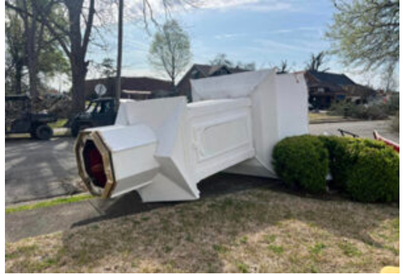
A steeple was blown off a building at First Baptist Church Rolling Fork, Miss., during tornadoes March 25. (Facebook Photo via BP)
