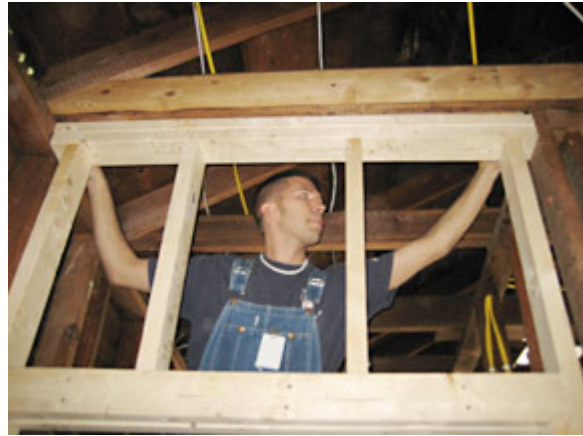
Ryan Plesko from First Baptist Church in College Station installs an interior frame.
