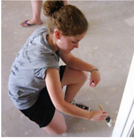
Bethany Elmore, a freshman at HPU, paints the trim on a home in Cross Plains that was damaged by the wildfires that hit in December 2005.
