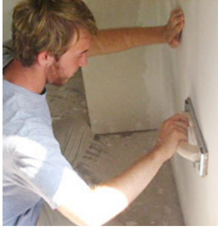
Josh Rhodes, a transfer student at HPU, helps with the dry walling in a home that was recently built in Cross Plains.
