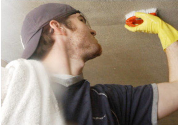
A Cameron University volunteer scrubs the ceiling of a Ringgold home that sustained substantial smoke damage.
